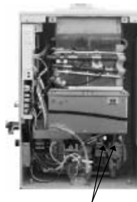
Manifold pressure taps.
